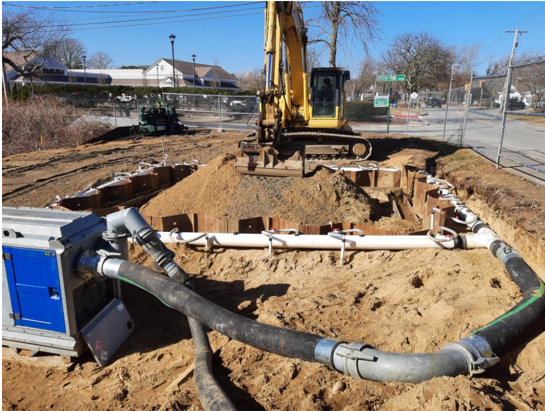
Groundwater Pumping System
