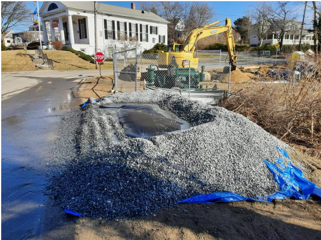
Clean Groundwater Discharge
